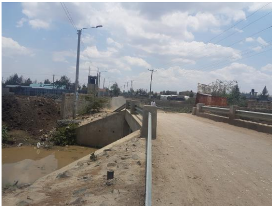
Part of the access road to the railway station that will be upgraded
